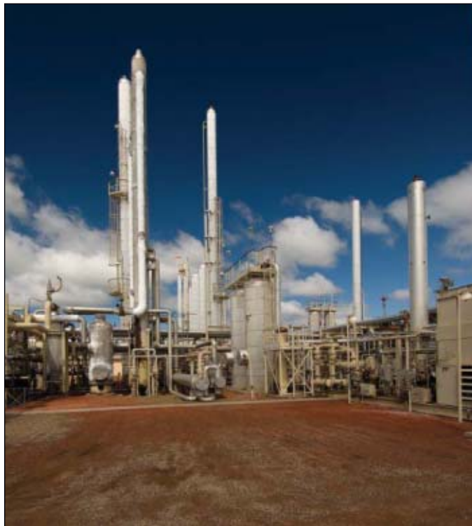
The Grasslands natural gas processing plant in McKenzie County, ND, is undergoing a $30 million expansion that will increase capacity by about 60% to 100 MMcfd. This plant is owned and operated by Bear Paw Energy LLC, a wholly owned subsidiary of Oneok Partners LP and is the partnership's largest natural gas plant in the Williston basin. (photograph from Oneok Partners by Rick Ayre)
